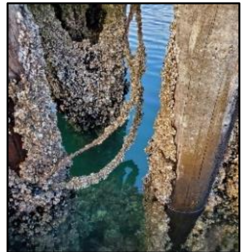
WIDESPREAD BREAKWATER COMPONENT FAILURE
